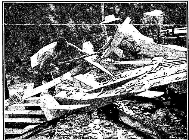
CARPENTERS WORKING ON ONE OF THE CURVED CORNERS OF THE ADMINISTRATION BUILDING
